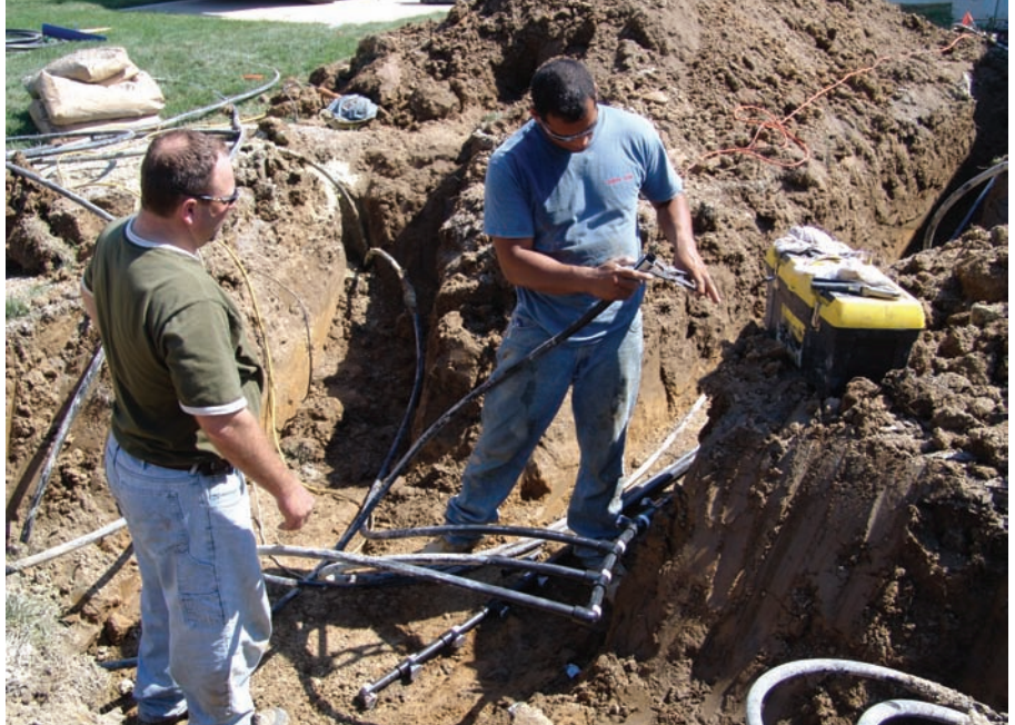
▲ The soil consistency and climate of a geothermal system’s installation plays a significant role in both how the system is designed and the size of the loop that will be necessary to transfer heat.
